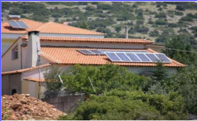
Solar Panel : Residence
